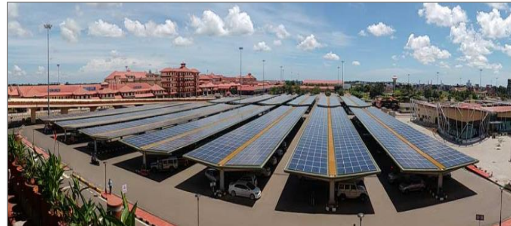
2.67 MW Carport installation at Cochin International Airport
