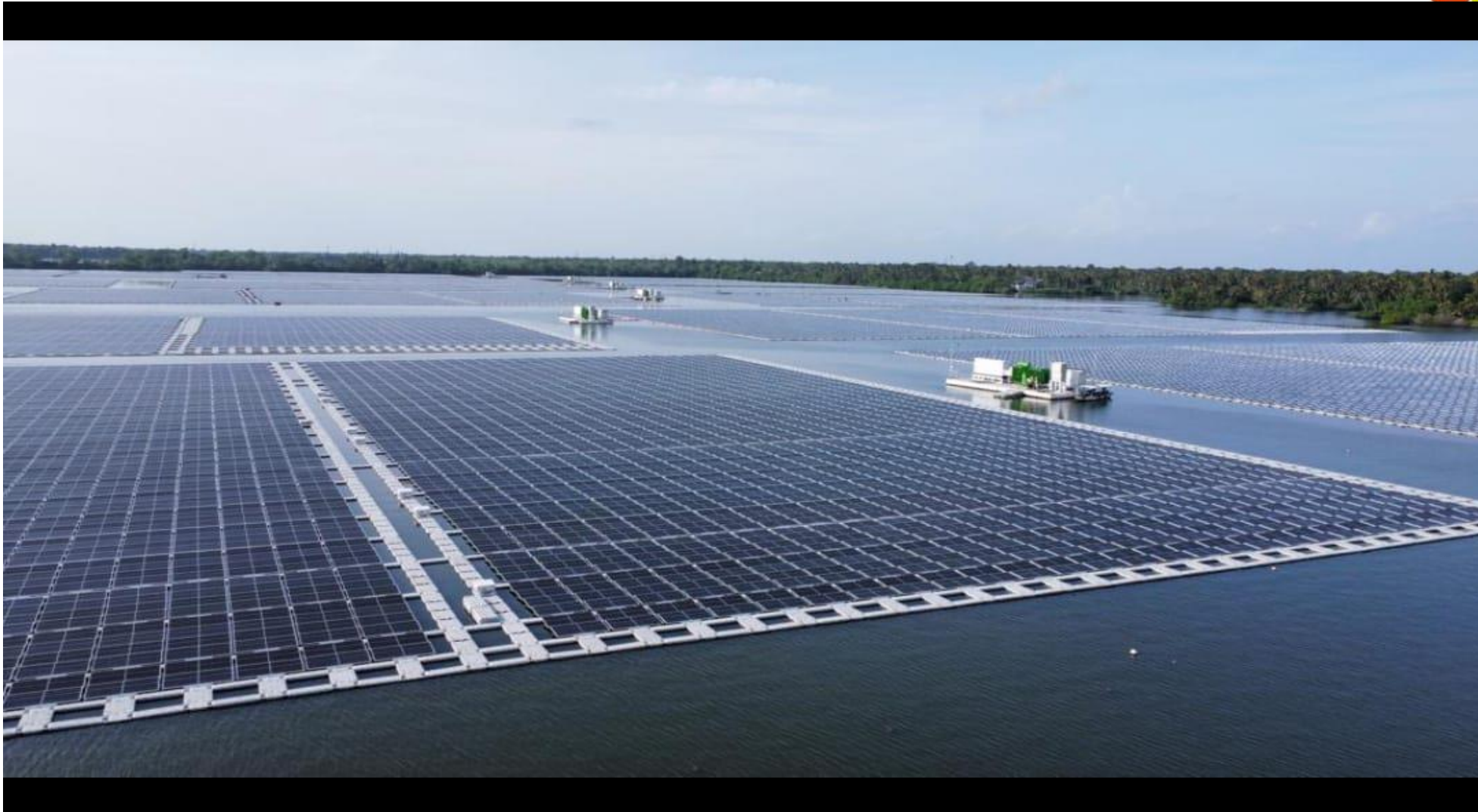
NTPC Kayamkulam – 70 MW
