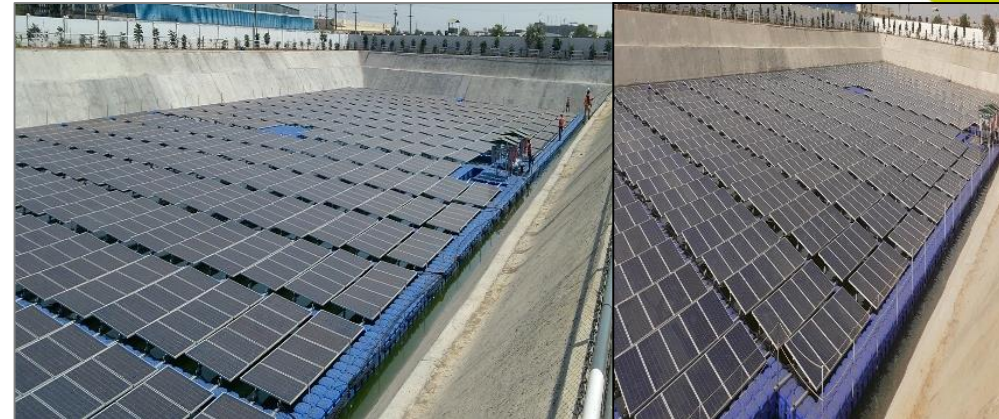
First Floating Solar System built on twin ponds with a capacity of 1.4MWp at Tata Chemicals, Nellore
